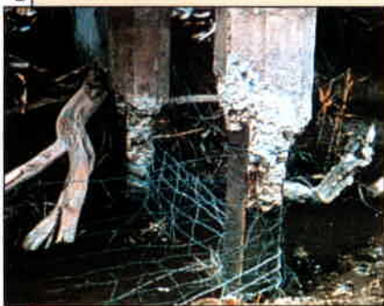
Concrete has deteriorated due to sulfate attack.
